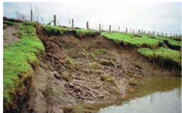
Example of riverbank erosion
