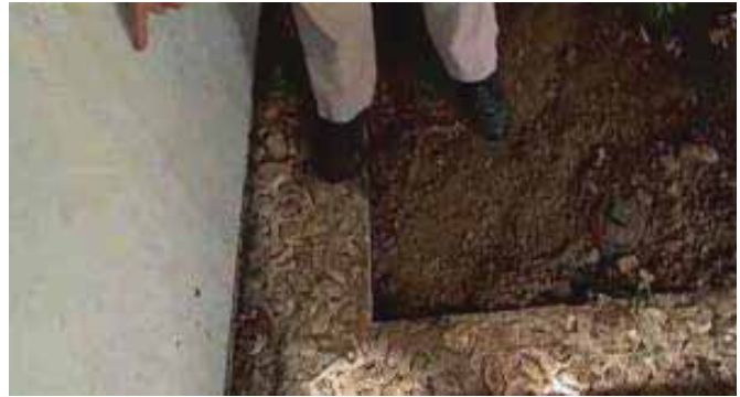
Homeowner Kent Affolter points to the end of his home's sewer line.
